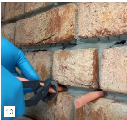
10 After applying the injection, the capillary rods remain in the masonry. Protruding ends are pulled out and cut off.
