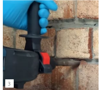
3 Drill horizontal holes (14 mm diameter) according to the table overleaf in the lowest horizontal joint with a depth of 5 cm less than the thickness of the masonry.
